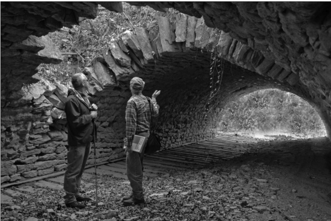
Mick Wilz and bridge expert Dr. James Cooper examine the hole in the Butler Run Aqueduct and discuss steps toward temporary repairs and possible restoration.
